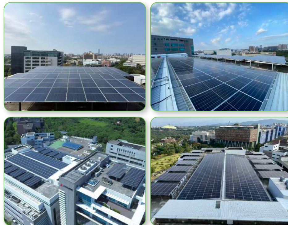
▲ Solar Photovoltaic Power Plant Installed on Headquarters Rooftop
